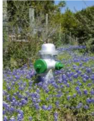
Here is a fire hydrant with a flow of 1,000-1,499 gallons per minute (GPM)
