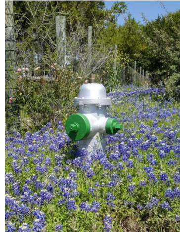
Here is a fire hydrant with a flow of 1,000-1,499 gallons per minute (GPM)
